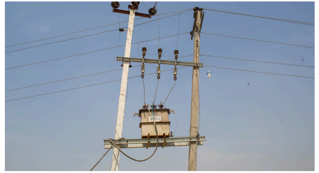
A grid connected pilot site in Nepal. (Photo: Nabin Baral for IWMI)
