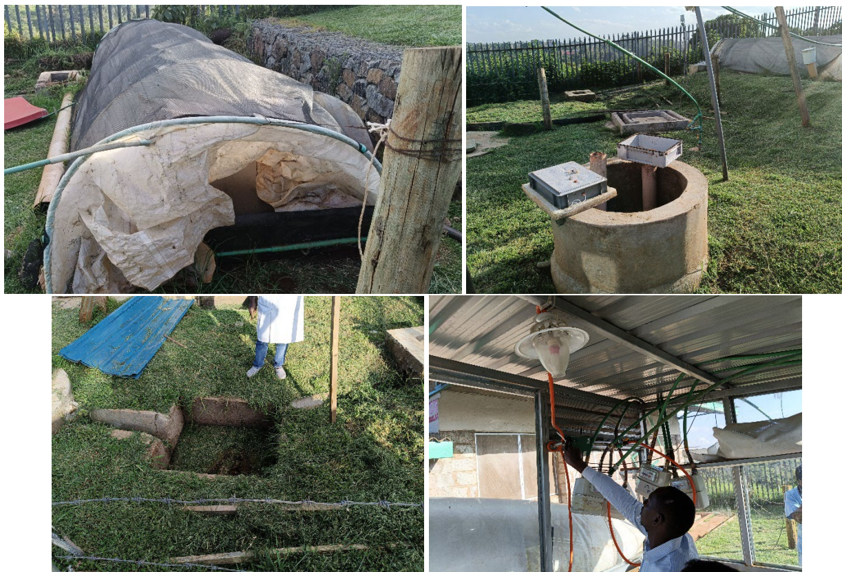
Biogas structure for bio-slurry and methane capture.
