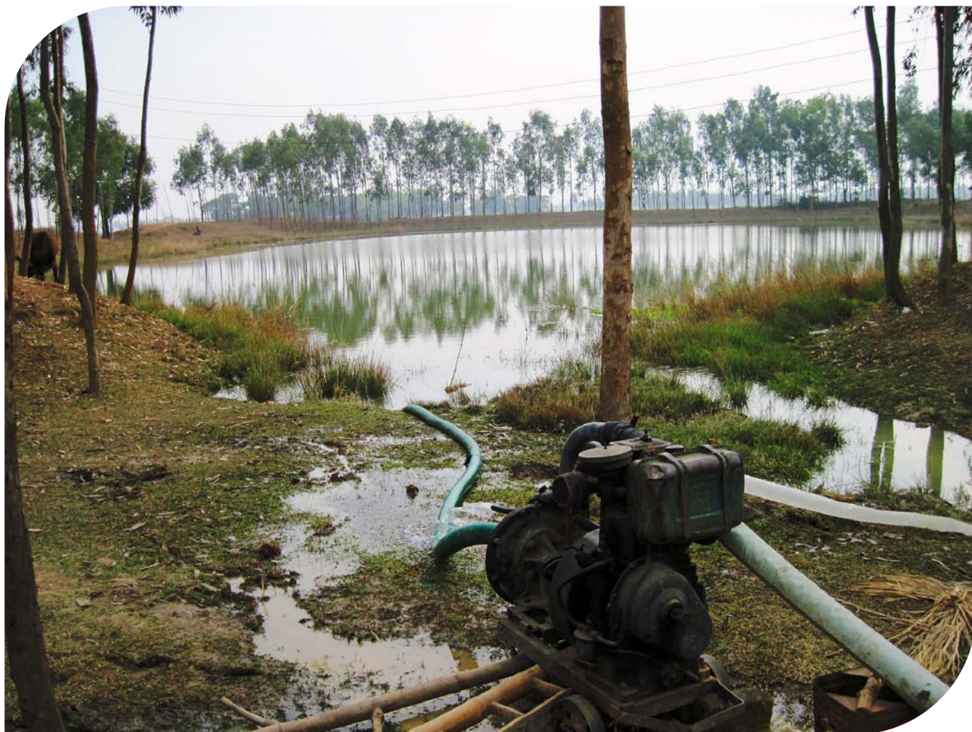
Electric pump that supplies groundwater to a farm in West Bengal (IWMI)
