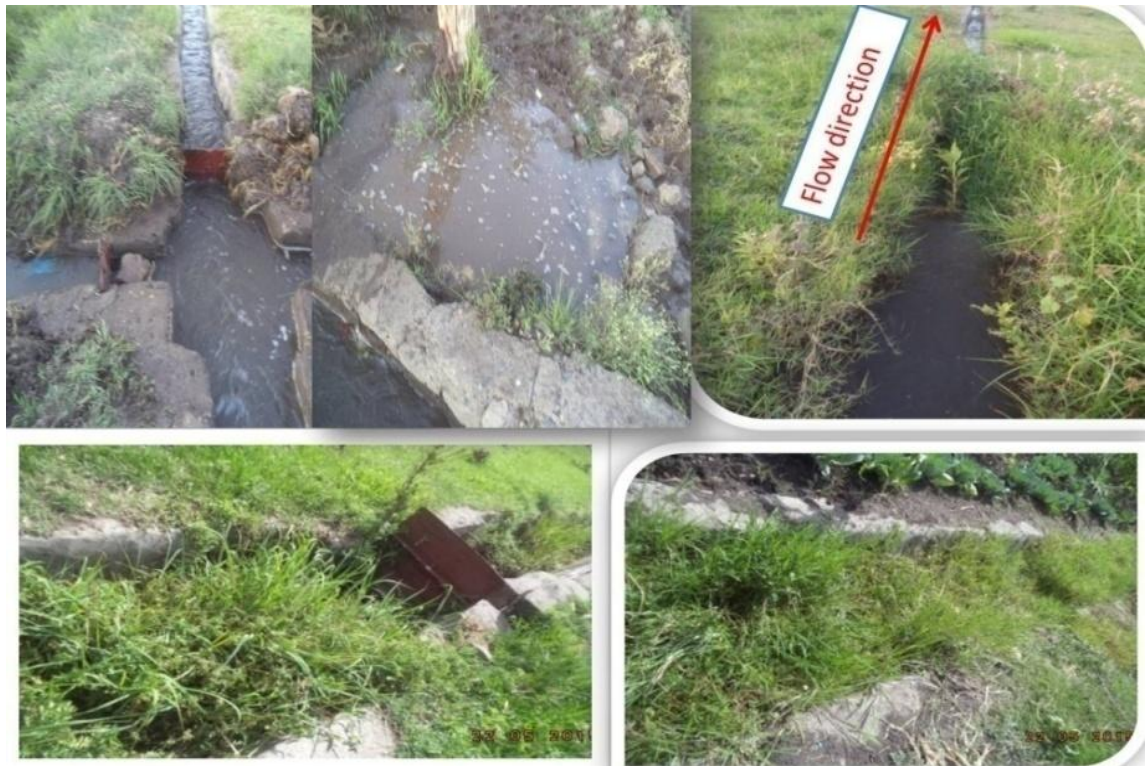
Figure 4.11: Secondary canals (silted, buried and over topped) at Jari SSI
