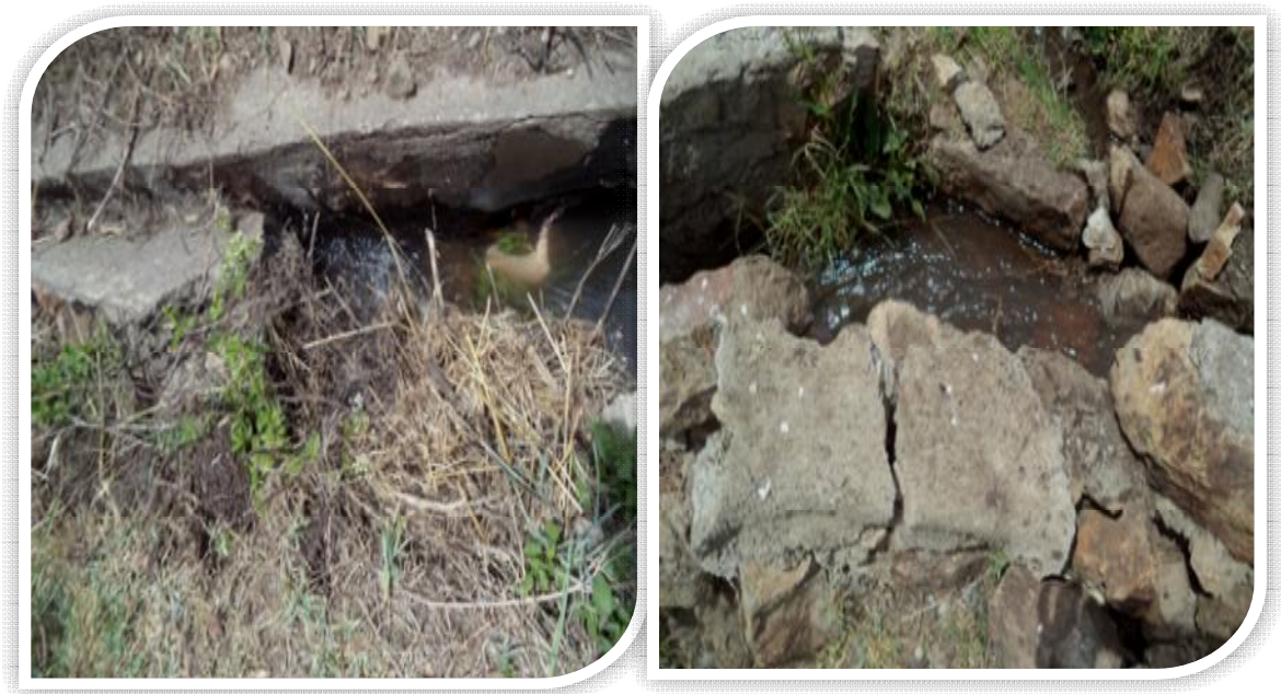
Figure 4.10: Cracked and fractured secondary canals at Aloma
