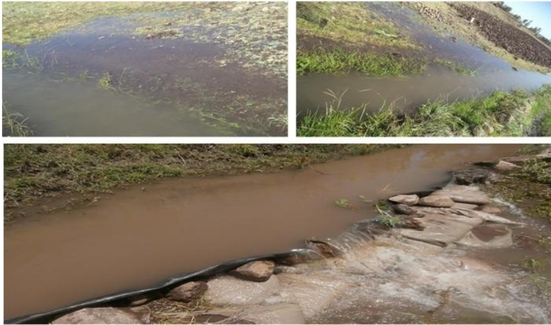
Appendix figure 7: Main canal water losses at Aloma SSI schemes (on earthen canal)
