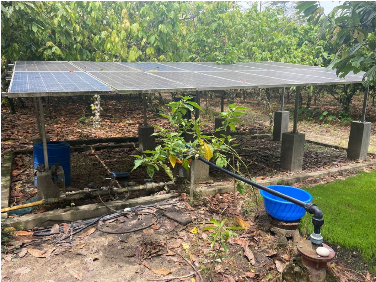
Figure 2. Example of a COCOBOD-installed solar-powered irrigation system located at Assin Fosu, Ghana
