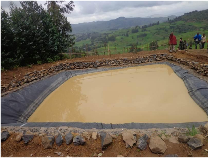
Figure 5. Water harvesting dam to irrigate and grow high value crops (photo credit: Kindu Mekonnen, ILRI)
