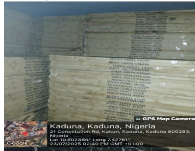
Exulted solar store room
