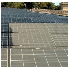
(E) Dust Accumulation
