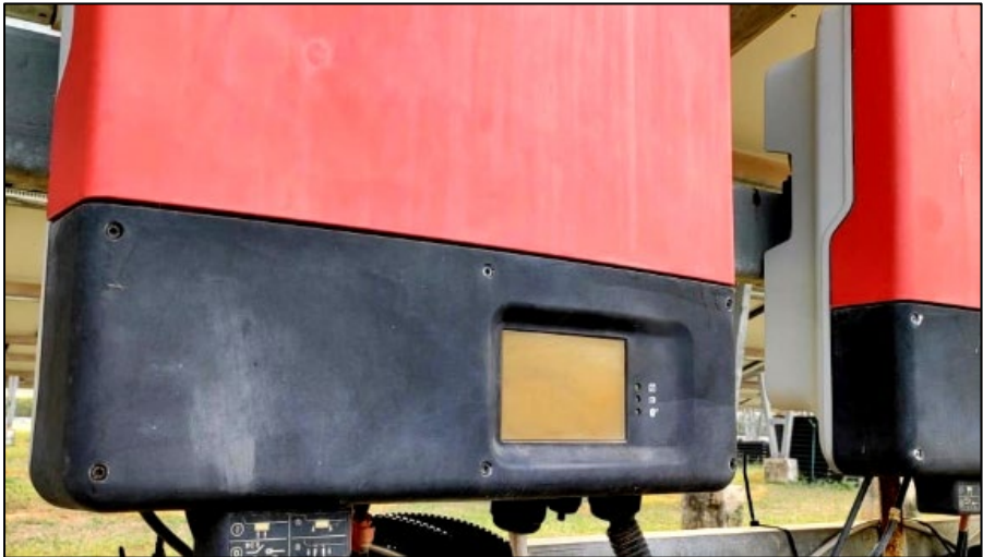
Figure 12. A grid-tied inverter for converting DC to AC photo: GERMI
