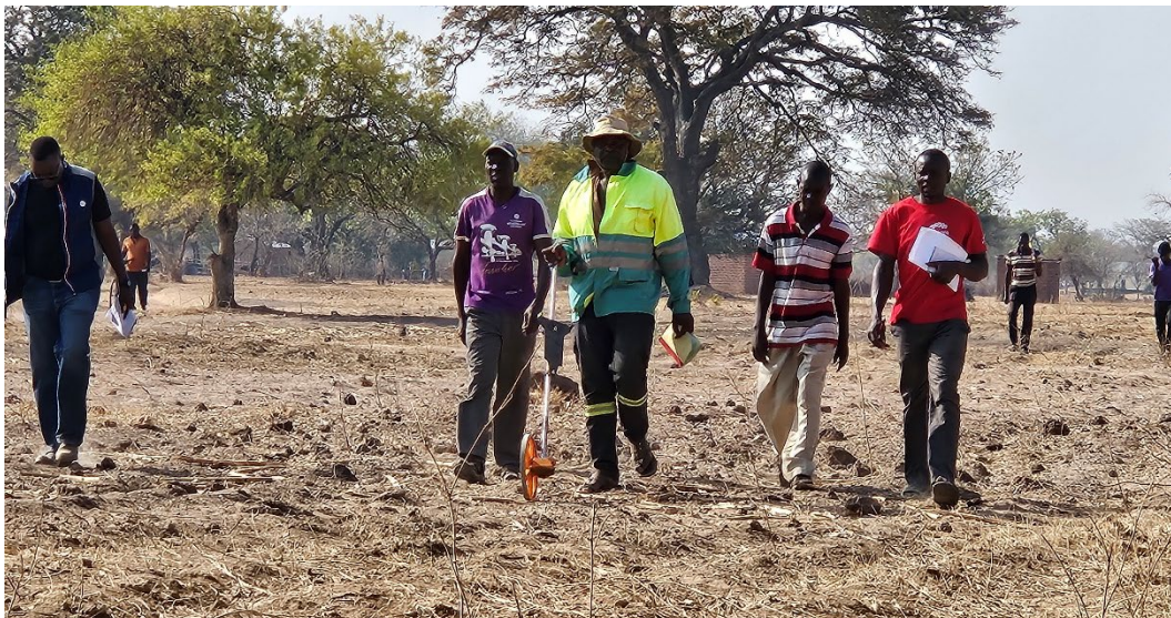
Figure 7. The team conducting a physical mapping exercise of sites to lay pipes and water access points (photo: Carol Mweemba 2025)
