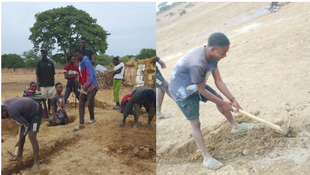
Figure 11. Men in Hanzila community digging trenches for laying water pipes (photo: Miyoba 2025)
