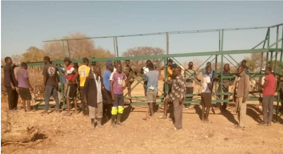
Figure 10. Men in Hanzila community attempting to place in position the tank stand (photo: Miyoba 2025)
