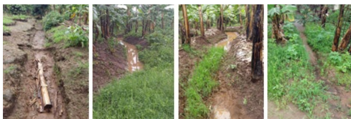
Figure 15: IRWH structures almost disappearing due to poor or lack of maintenance
