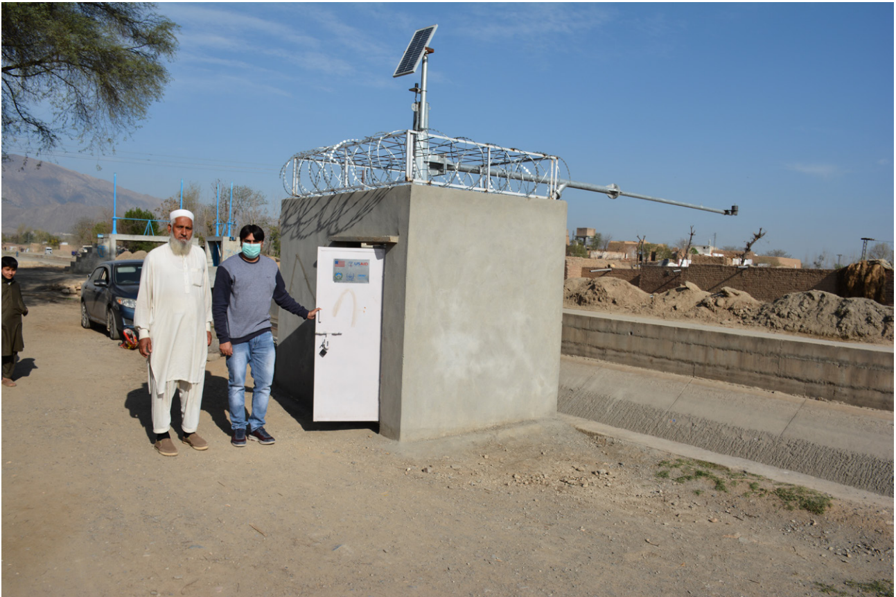
Figure 2. Indus Telemetry installation at Warsak Gravity Canal. (photo: Kashif Hussain/IWMI)
