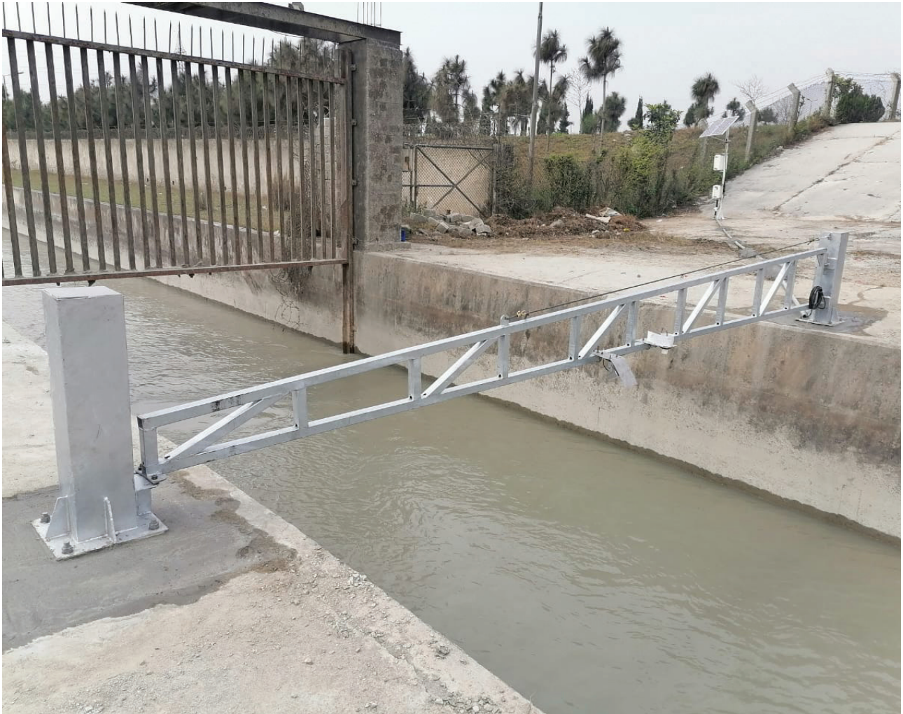
Figure 1. Indus Telemetry installation at Pehur High Level Canal. (photo: Muhammad Tousif Bhatti/IWMI)
