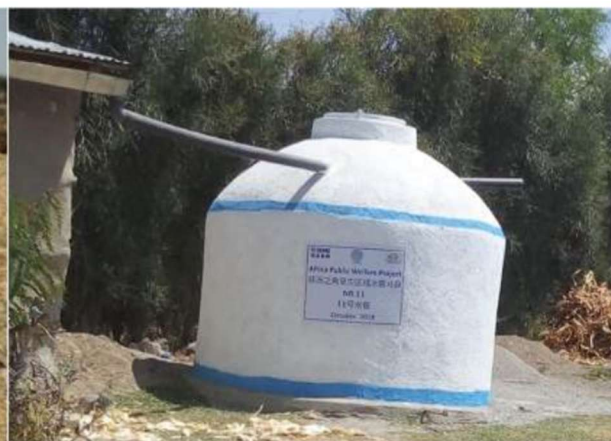
Above ground WHS, Adami Tulu
