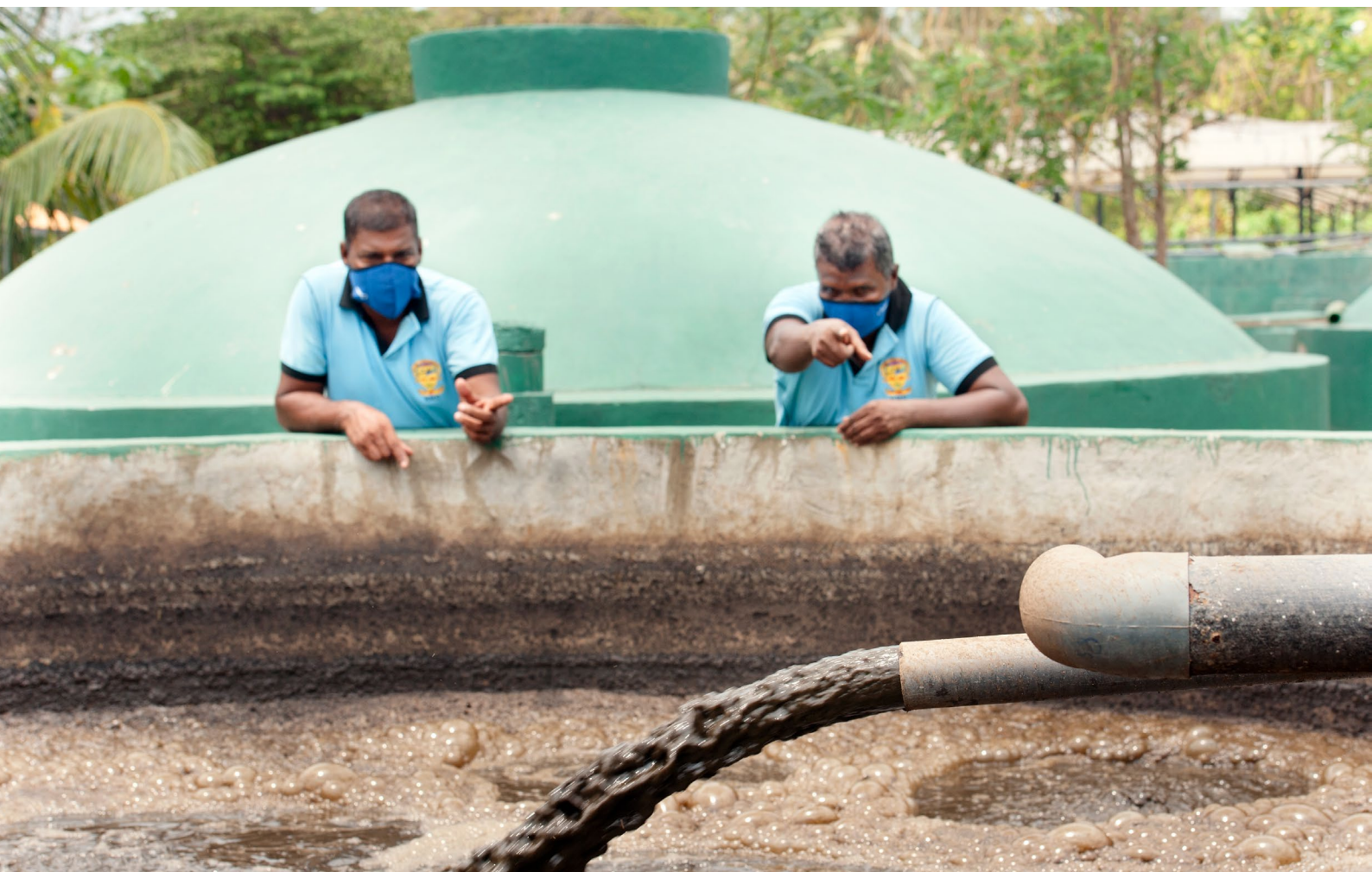
View of inside of Bio Gas Tanks (Fecal Sludge Treatment Unit), Sri Lanka. Photography by Hamish John Appleby / IWMI
