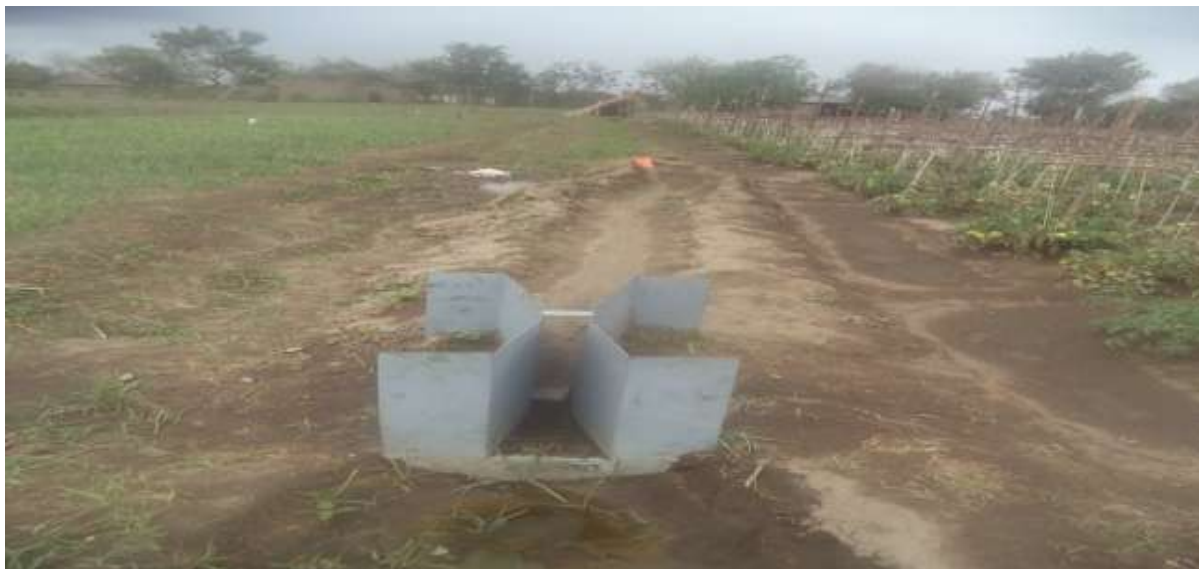
Appendix Figure 9. Parshall flume installed for discharge measurement
