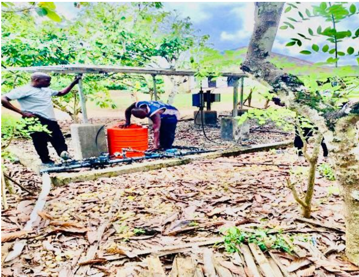
Figure 7. Solar Irrigation facility (photo: Daniel Agyemang/IWMI)
