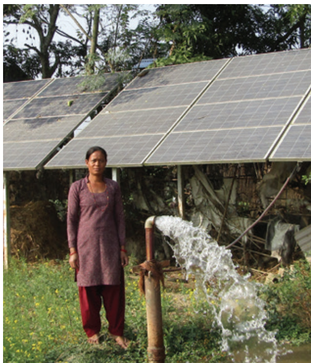
Solar-based irrigation system at Agyauli, Nawalpur
