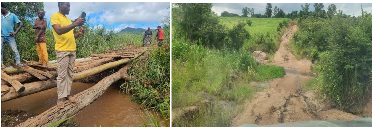
Figure 7. Example of poor road condition
