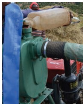
Step 2: Fill water at the right top of the pump until it is full (priming).
