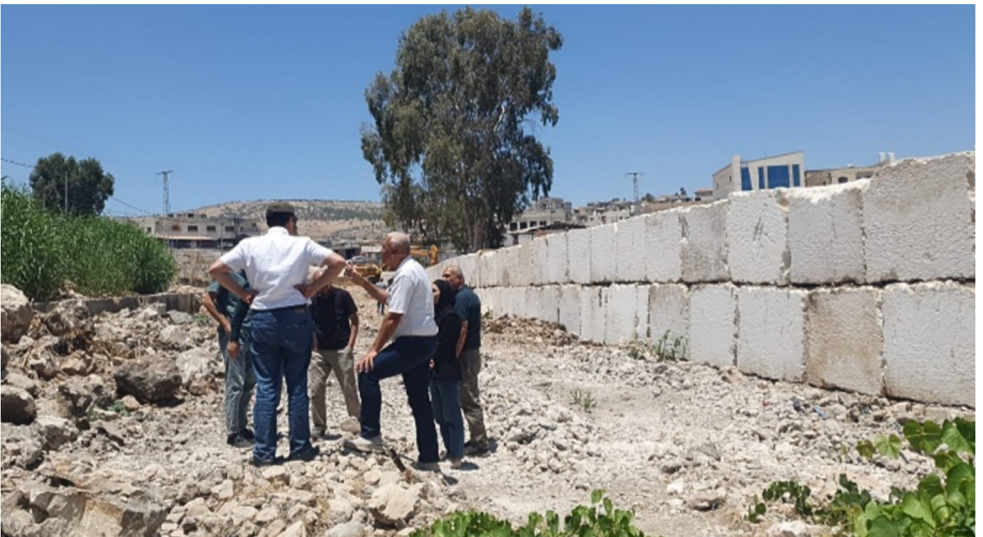
Ongoing works for Ain Fari'a and wadi channel rehabilitation (photo: Palestinian Hydrology Group [PHG])
