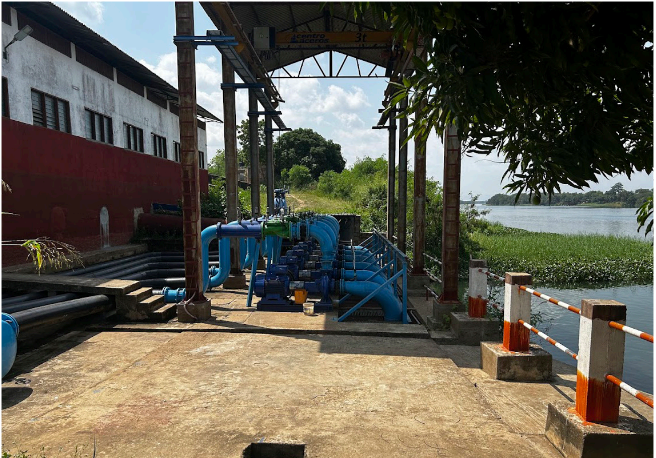
Figure 9. Installed water pumps at the Kpong irrigation scheme to abstract water from the Volta River. photo: Birhanu Zemadim/IWMI
