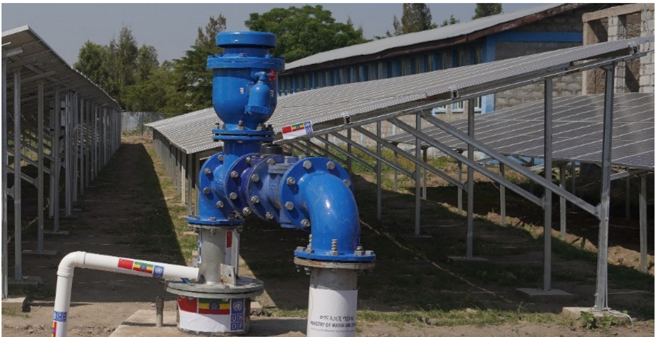
Figure 13. Solar-powered irrigation system in the Sidama region of Ethiopia.
