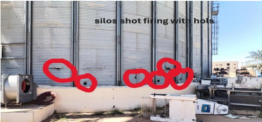
Image 1: Silo damage at wheat flour mill Factory 1, Khartoum North industrial area, March 2025
