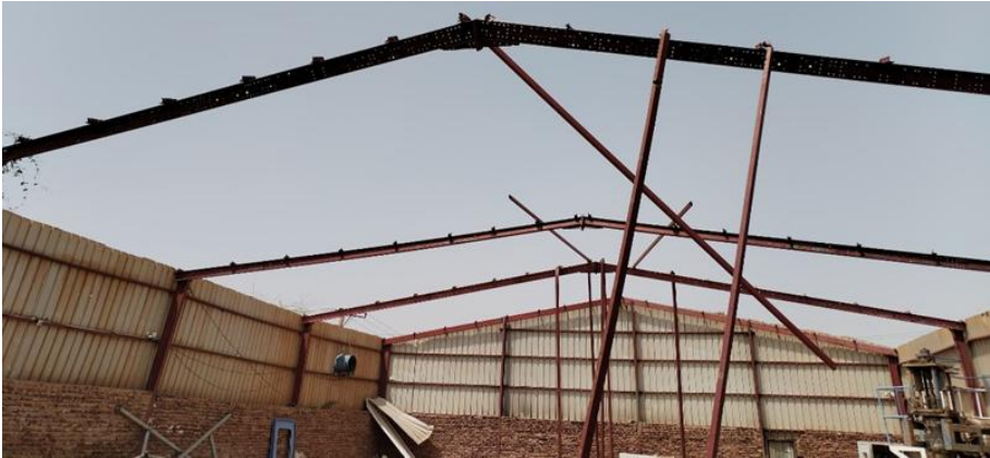
Image 7: Edible oil industry, theft of roof sheeting at edible oil factory, Khartoum North industrial area, March 2025
