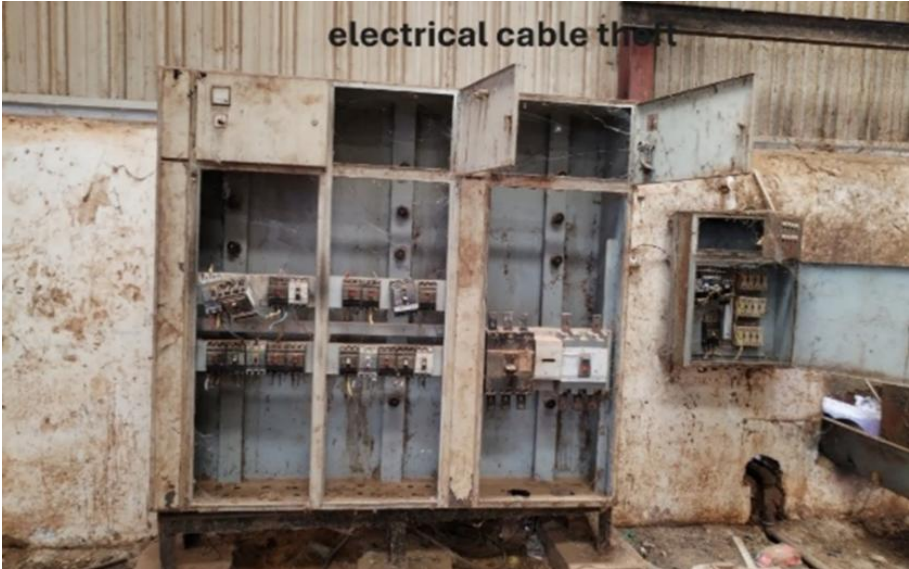
Image 5: Damaged electrical system panel, wheat flour mill Factory 1, Khartoum North industrial area, March 2025
