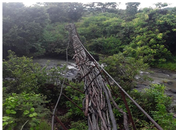
Fig. 2 Damage to Murozi Footbridge caused by Cyclone Ana in Ward 13, Nyanga District. Photograph by Vuyisile Ndlovu, Christian Aid
