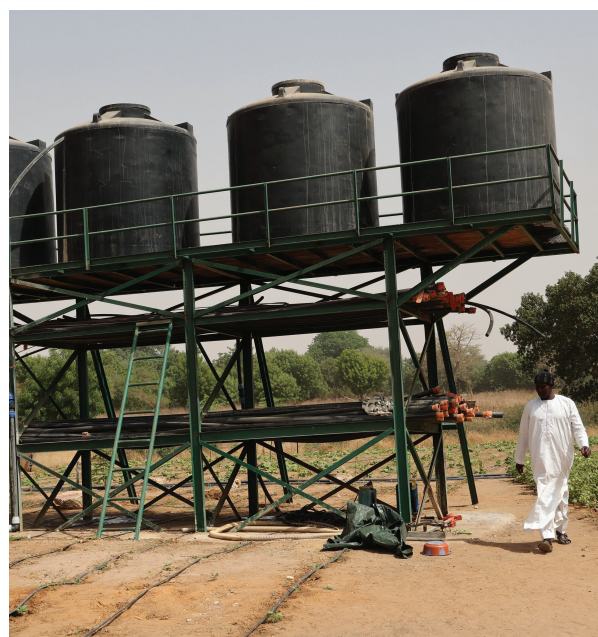
Field in Paaskoto, Kaolack Region, Sénégal, equipped with a drip irrigation system powered by solar panels, pumping water from both a well and a borehole. (photo: Xavier/Shutterstock).
